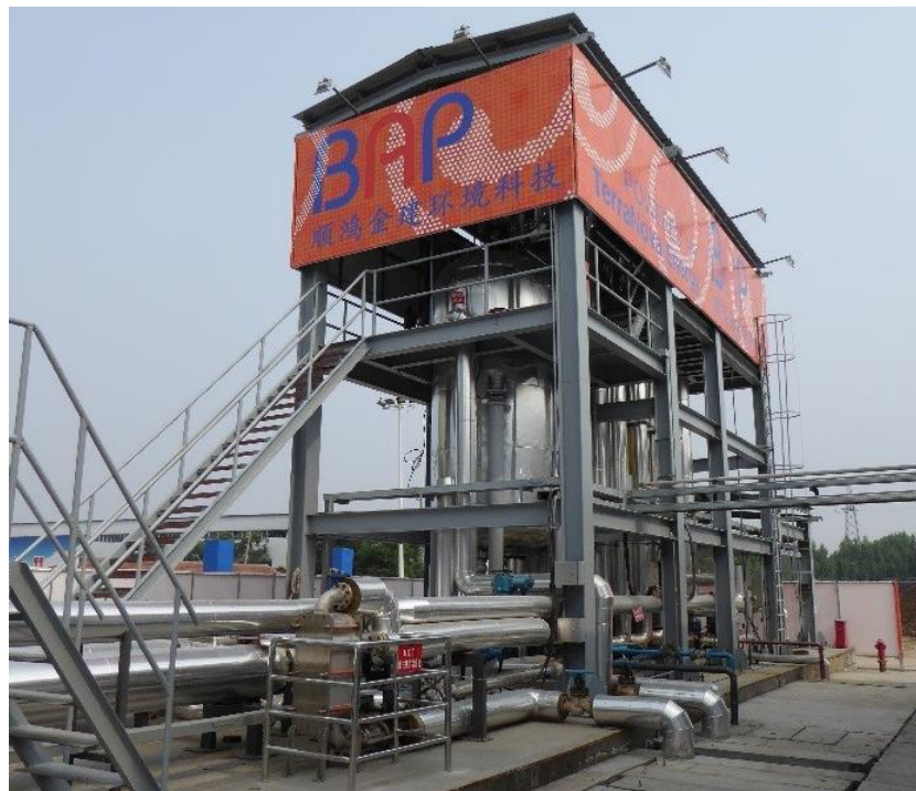
Abbildung 5.3: TerraNova® Ultra-Anlage in Jining, China [Holinger 2017]
